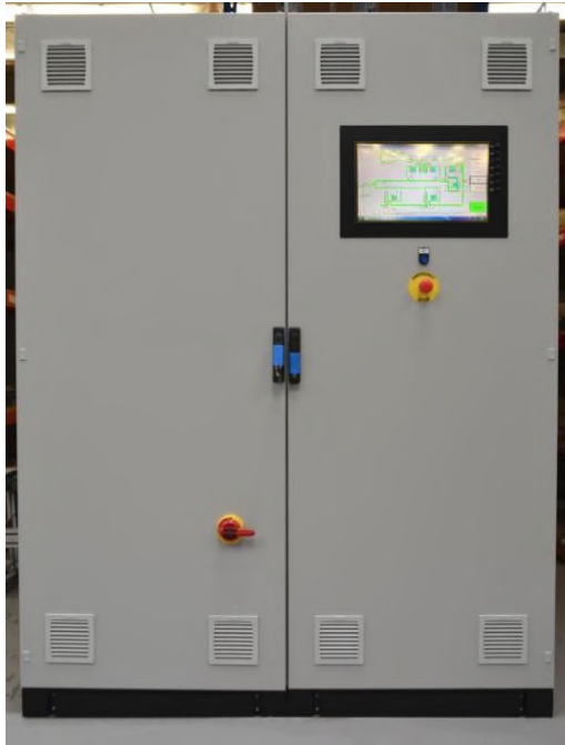
Control Panel with Touch Screen HMI
